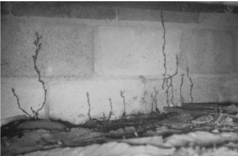
Figure 4. Termite tubes on the foundation of a structure.
